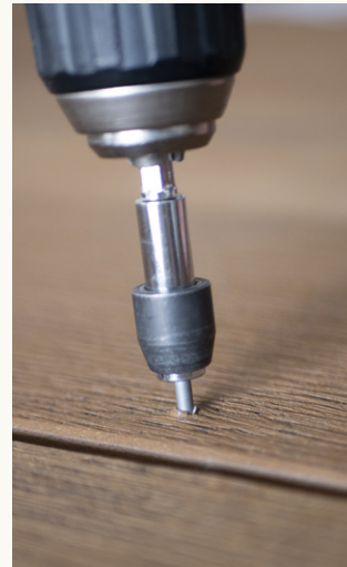
Screw driven below surface with drill; Lastane layer begins to compress around the fixing.
