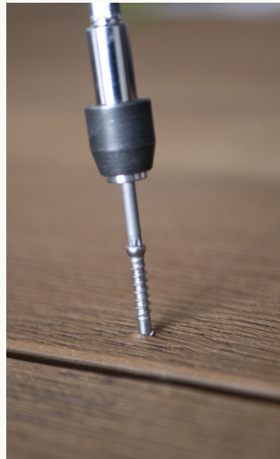
Screw aligned above board surface prior to installation using Durafix® screw and driver bit.
